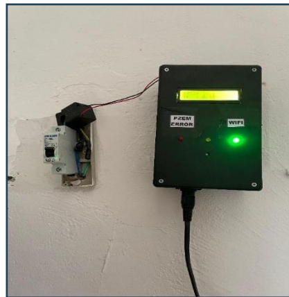
Figure 3 . Testing of kWh monitoring tools
